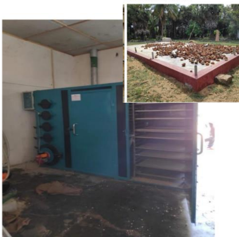
Above: MPCS Coconut Mill project Copra Drying Machine
